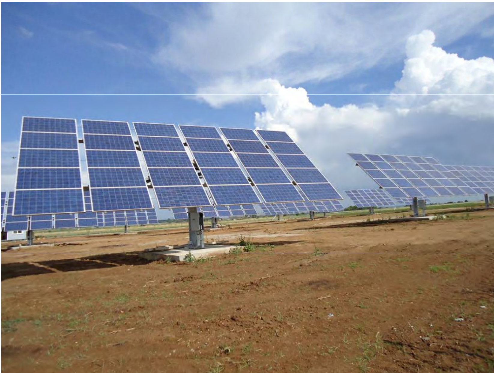
100kWp tracking system, Kilis
