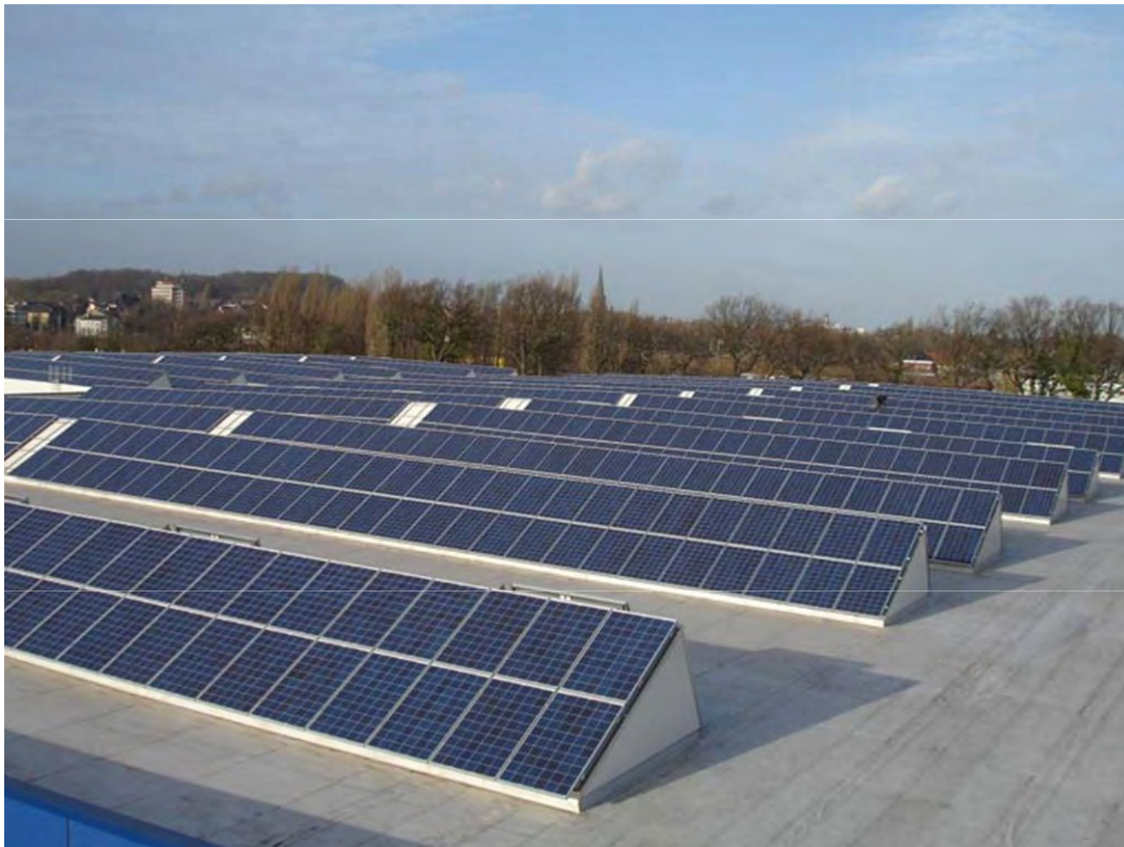
200kWp Industrial rooftop, Athens
