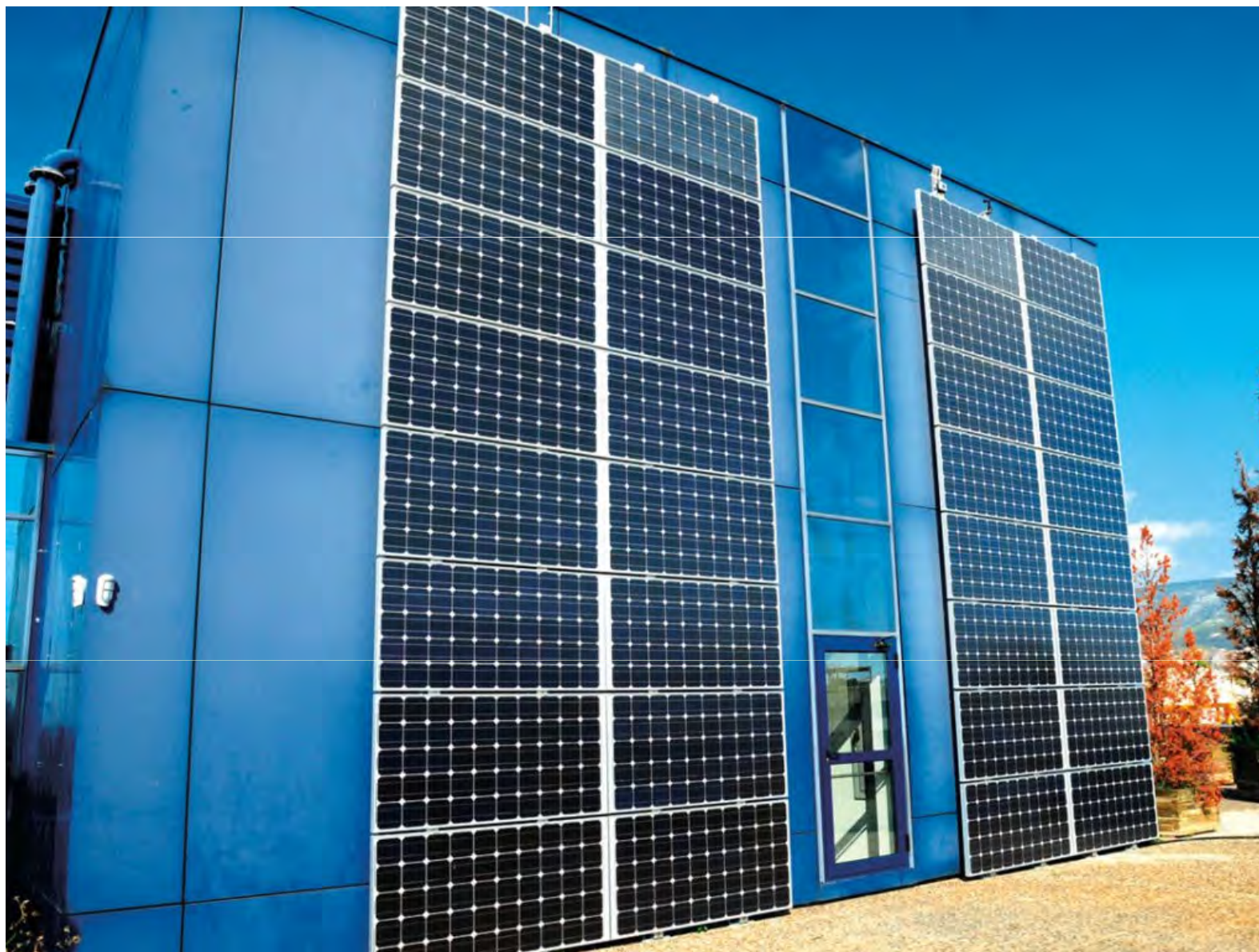
5kWp Façade, Athens
