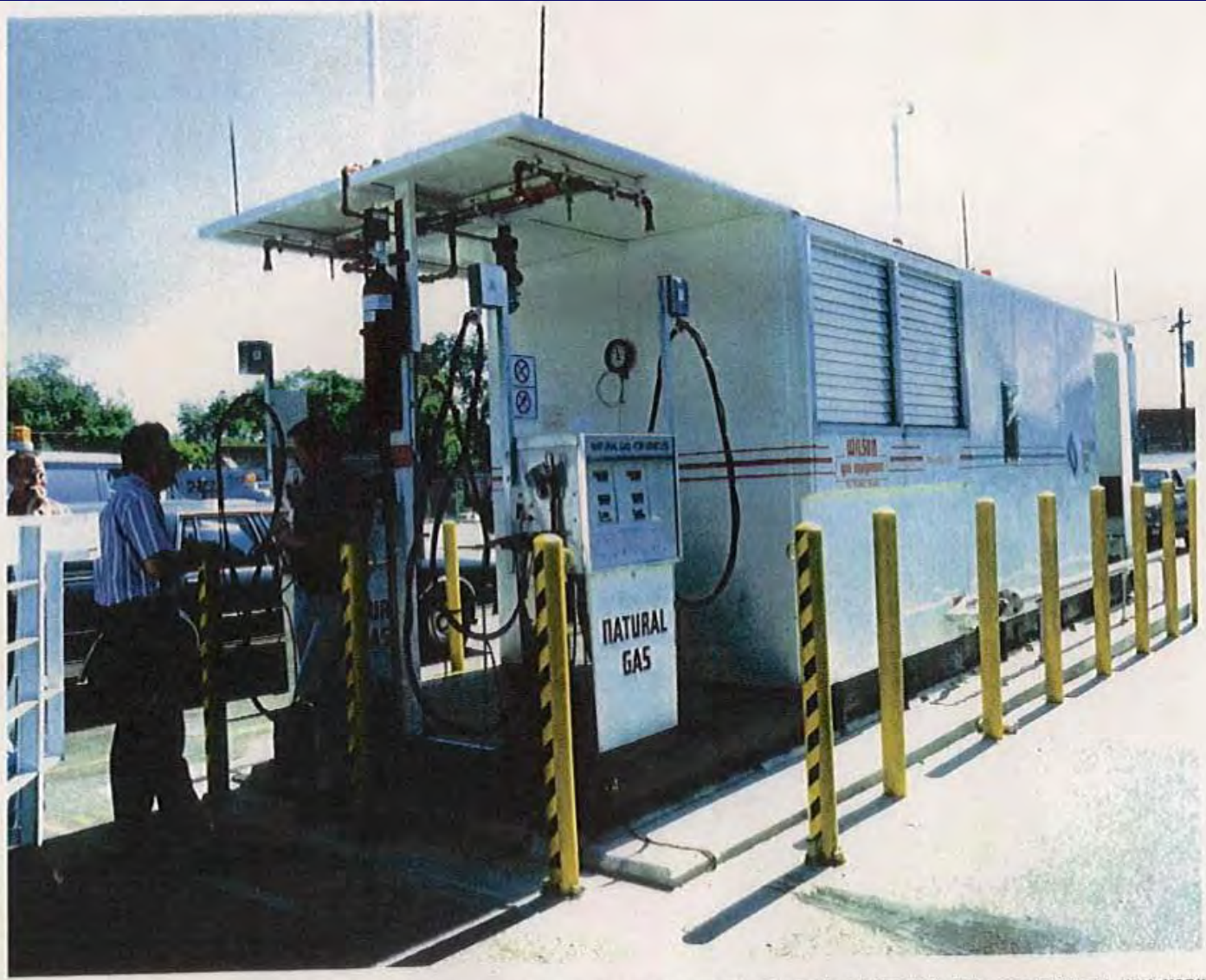
CNG UNIT AND DISPENSERS SUPPLIED BY NUOVO PIGNONE TO BROOKLYN UNION GAS FOR DEDICATED CNG STATION IN NEW YORK
