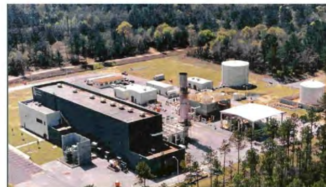
Alabama CAES plant – 110 MW 24 hr This facility uses a single large salt dome cavern of 560,000 m 3 , and is capable of storing 2.6 GWh of energy. Daily cycling for 1 or 2 periods, start to full load <15 mins
