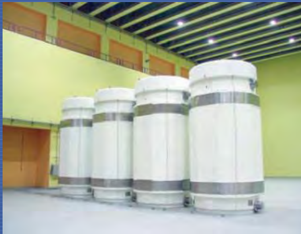
Dry storage casks
