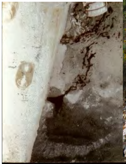
Loutra Kyllinis oil seep
